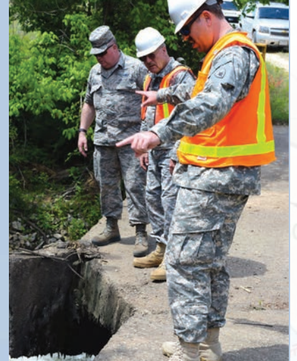
TEXAS STATE GUARD ENGINEERS trained on infrastructure assessment during annual training at Camp Swift, Bastrop, Texas, April 26-29, 2018. Engineers evaluated the structural integrity of key infrastructure elements such as bridges, buildings and a local waste water facility.
